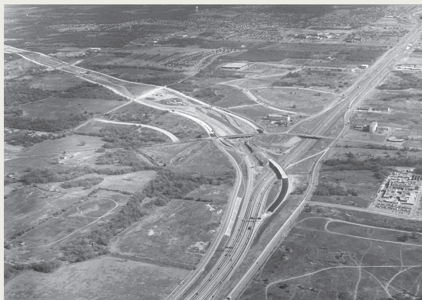
Figure 4-28. Aerial view of the Airport Freeway (SH 121) under construction in a predominantly undeveloped section of Fort Worth, looking east. Source: “Looking east on Airport Freeway with Highway 121 construction,” Fort Worth Star-Telegram Collection, University of Texas at Arlington Libraries Digital Gallery, 1979, accessed June 15, 2021, https://library.uta.edu/digitalgallery/img/10002802 .
