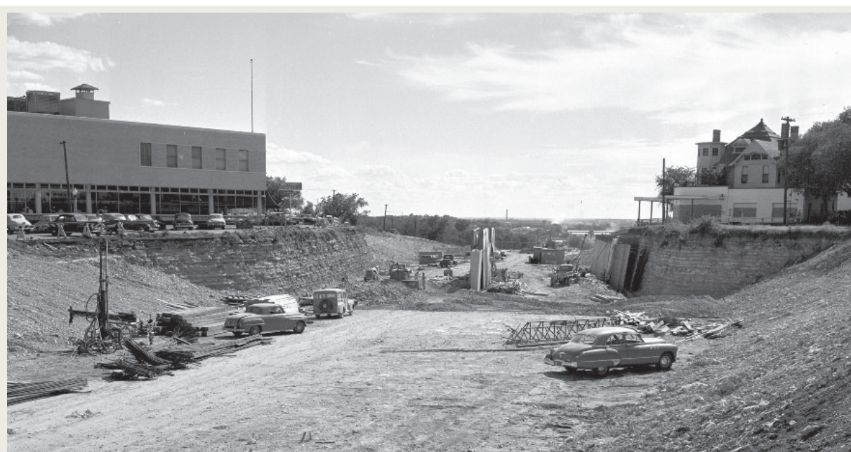
Figure 4-21. Construction of the East–West Freeway on the west side of downtown at Summit Avenue in 1951. Source: “Fort Worth’s East–West expressway under construction,” Fort Worth Star-Telegram Collection, University of Texas at Arlington Libraries Digital Gallery, 1951, accessed May 19, 2021, https://library.uta.edu/digitalgallery/img/20057102 .
