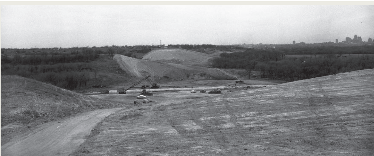
Figure 4-23. Construction of the Dallas–Fort Worth Turnpike between Oakland Boulevard and Beach Street in East Fort Worth. Source: “Construction of the Dallas-Fort Worth Turnpike between Oakland Boulevard and Beach Street on Fort Worth’s East Side,” Fort Worth Star-Telegram Collection, University of Texas at Arlington Libraries Digital Gallery, 1956, accessed June 15, 2021, https://library.uta.edu/digitalgallery/img/20057134 .
