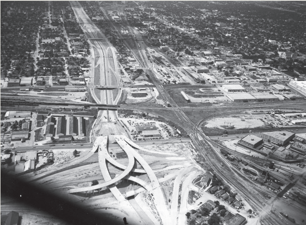
Figure 4-24. Aerial view of the construction of the Dallas–Fort Worth Turnpike interchange at Lancaster Avenue near downtown in the late 1950s, looking south. Source: “Aerial view of the new Dallas-Fort Worth Turnpike interchange at Lancaster Avenue, Fort Worth, Texas,” Fort Worth Star-Telegram Collection, University of Texas at Arlington Libraries Digital Gallery, 1957, accessed June 15, 2021, https://library.uta.edu/digitalgallery/img/20059613 .
