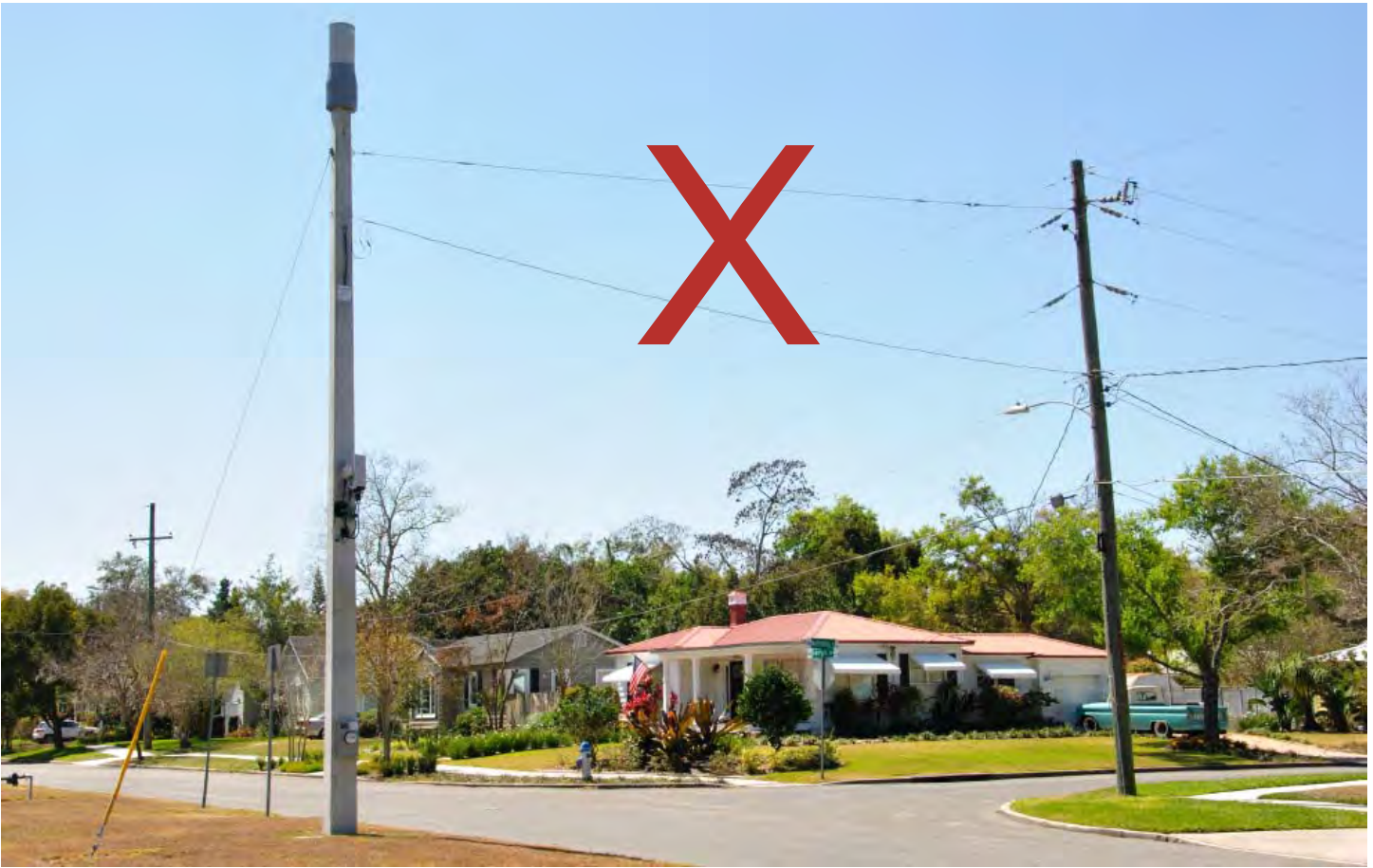
Exhibit 7- Aerial power and fiber connections are not be permitted. They create additional visual clutter and may require extra tension and structural support.
