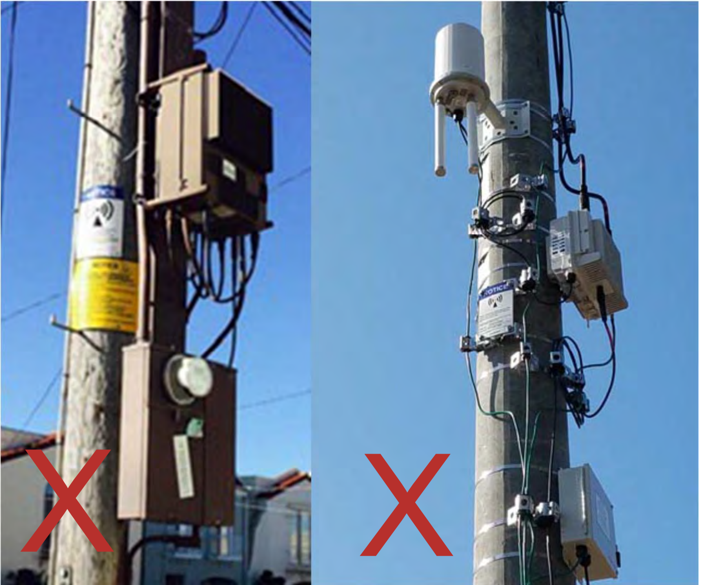
Exhibit 17– The cabling that is cluttered & tangled. Excess loose cabling, excess decals/ stickers, and cluttered appearance of equipment cabinets is not allowed. Repetitive, and highly visible RF warning stickers, and equipment manufacturer decals located near bottom of pole and visible to pedestrians are not allowed. The presence of multiple stickers and manufacturer logos, which should be removed or painted over.
