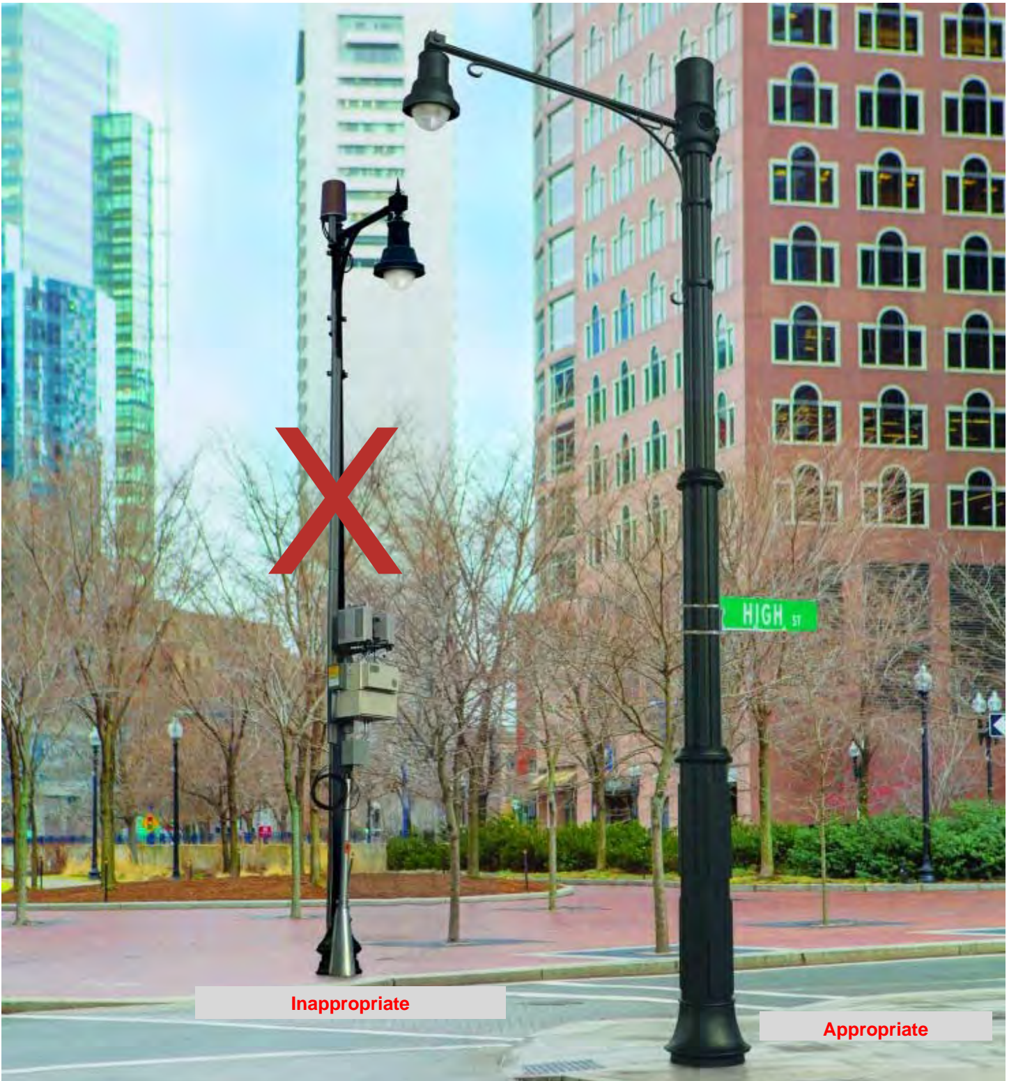
Exhibit 9– The Pole on the right the Wireless Facility is mounted in an inconspicuous location and painted to match. The Pole on the left the Wireless Facility is a different color than the pole and there is exposed conduit.
