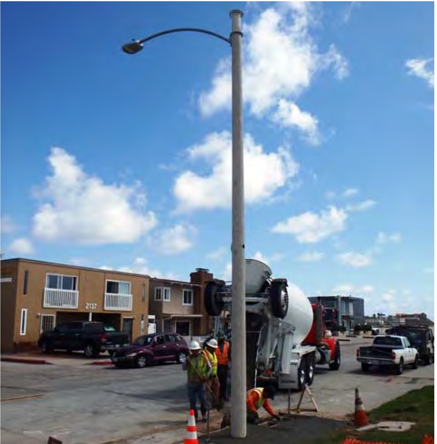
Exhibit 10- Exposed wiring is prohibited. Above the electric meter and disconnect switch, all conduit and wiring shall be located inside the pole. All equipment is located inside the pole and avoids creating physical or visual obstruction to pedestrian and vehicular traffic.
