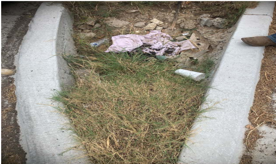
Source: Incomplete backfilling of a curb at 615 NW 25TH and Prospect, observed by Internal Audit on 07/29/2020
