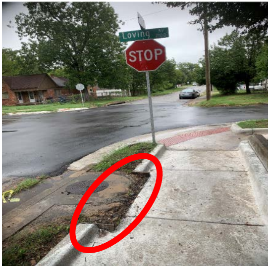
Source: Auditor photograph (Trip hazard Loving Avenue)
