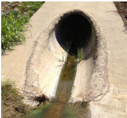
Dry weather discharge.
