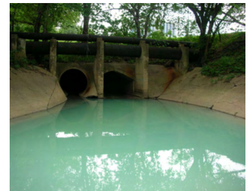
Complaint received of discolored water.
