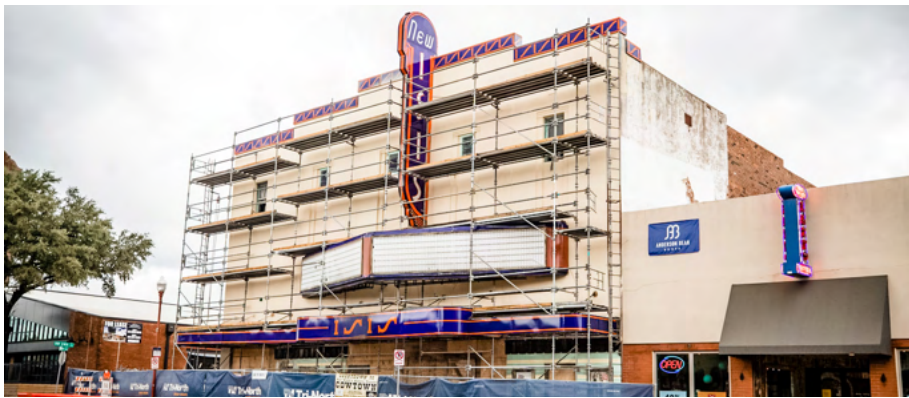
The New Isis Theater, which had sat vacant for decades prior to the adoption of the Stockyards Form-Based Code, has been undergoing rehabilitation since 2018. (Source: City of Fort Worth, Development Services Department, 2021.)
