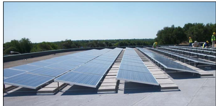
Solar panels were installed at the City's trash and recycling drop-off station on Hemphill Road in February 2011 (above) and at the Southwest Regional Library in June 2011 (below). (Source: Transportation and Public Works Department, 2011.)
