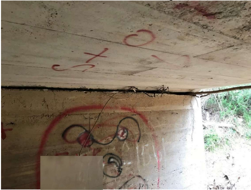
Photo 3: Westside of intermediate support has sunk several inches and not supporting the roadway above
