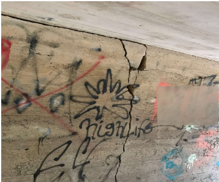
Photo 2: Close up of large crack in middle of intermediate bridge support indicating movement or erosion of foundation
