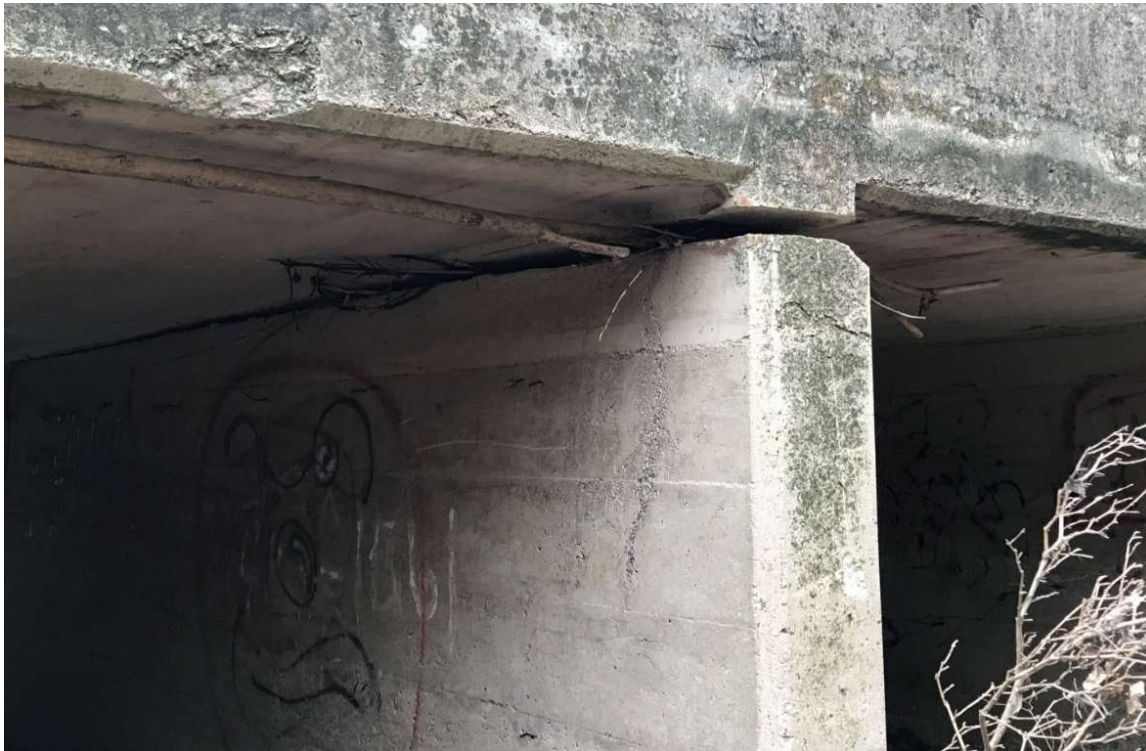
Photo 4: Close up of intermediate support settlement
