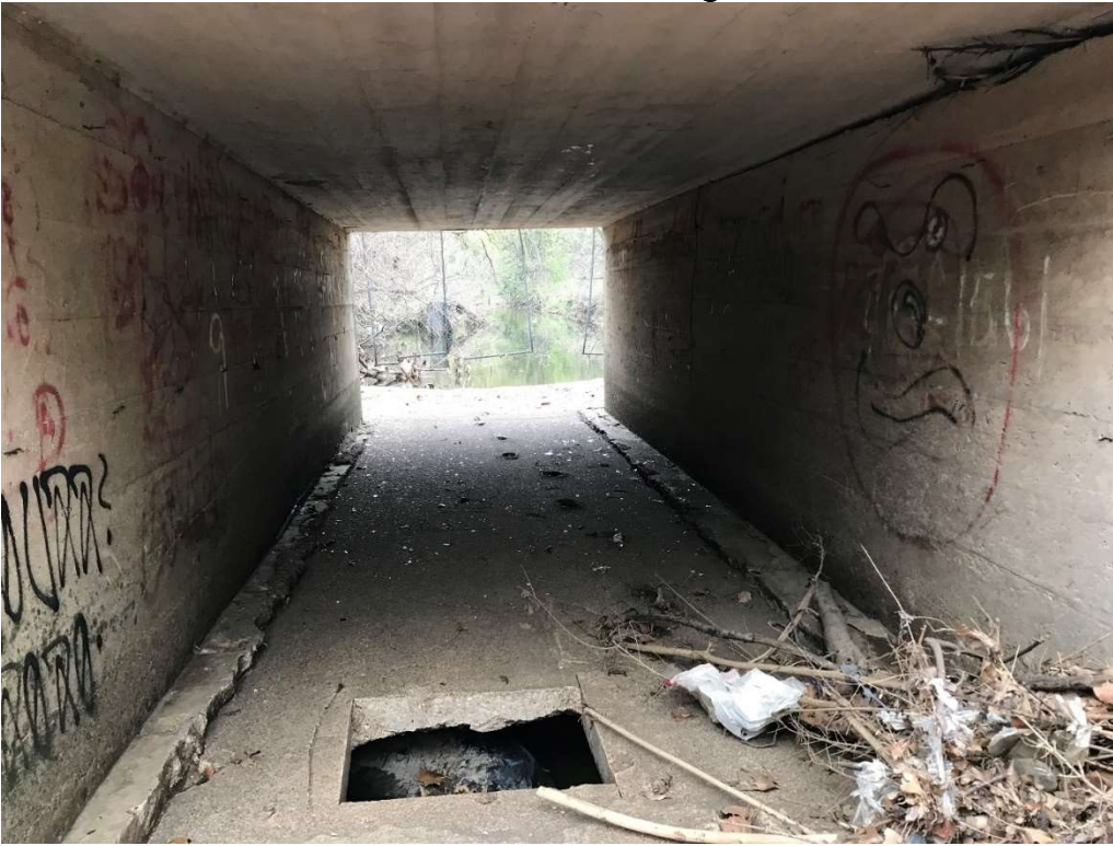
Photo 5: Hole in culvert floor allowing water to erode below
