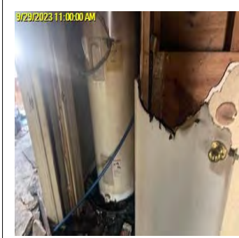
Comp/Insp Date: 9/29/2023 Damage Photo
