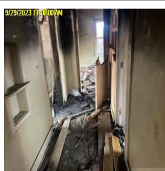
Comp/Insp Date: 9/29/2023 Damage Photo
