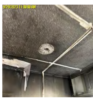
Comp/Insp Date: 9/29/2023 Damage Photo
