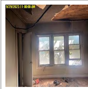
Comp/Insp Date: 9/29/2023 Damage Photo
