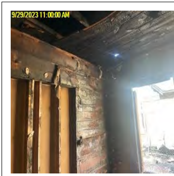
Comp/Insp Date: 9/29/2023 Damage Photo
