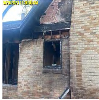
Comp/Insp Date: 9/29/2023 Damage Photo
