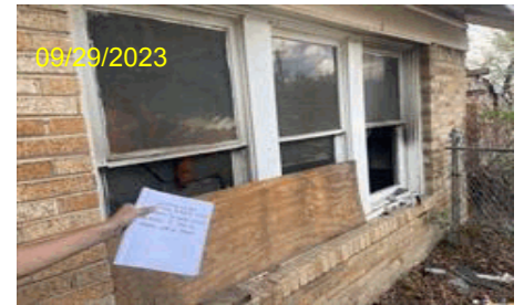
Image Type:Completion Before Photo Address:4433 Virginia Ln City,State Zip:Forth Worth, TX 76103 Line Item Desc:Photos
