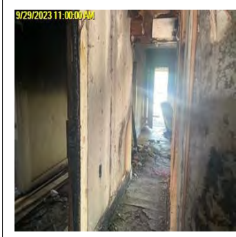
Comp/Insp Date: 9/29/2023 Damage Photo
