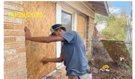
Image Type:Completion During Photo Address:4433 Virginia Ln City,State Zip:Forth Worth, TX 76103 Line Item Desc:Photos
