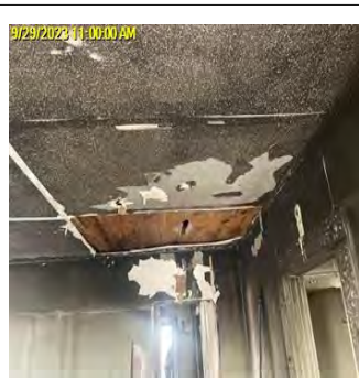
Comp/Insp Date: 9/29/2023 Ceiling - Interior
