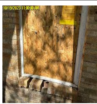
Comp/Insp Date: 10/19/2023 Work Not Needed Board All Accessible Openings
