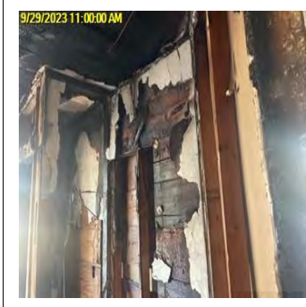
Comp/Insp Date: 9/29/2023 Damage Photo
