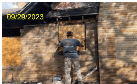
Image Type:Completion During Photo Address:4433 Virginia Ln City,State Zip:Forth Worth, TX 76103 Line Item Desc:Photos
