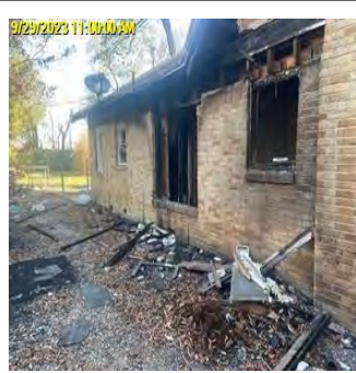
Comp/Insp Date: 9/29/2023 Damage Photo
