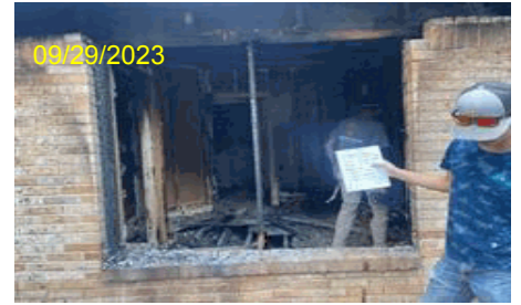
Image Type:Completion Before Photo Address:4433 Virginia Ln City,State Zip:Forth Worth, TX 76103 Line Item Desc:Photos
