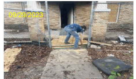
Image Type:Completion During Photo Address:4433 Virginia Ln City,State Zip:Forth Worth, TX 76103 Line Item Desc:Photos
