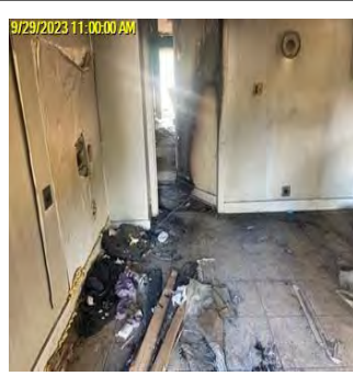
Comp/Insp Date: 9/29/2023 Damage Photo
