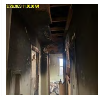
Comp/Insp Date: 9/29/2023 Damage Photo
