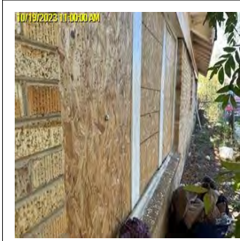
Comp/Insp Date: 10/19/2023 Work Not Needed Board All Accessible Openings
