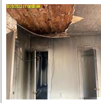
Comp/Insp Date: 9/29/2023 Damage Photo
