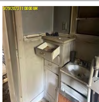
Comp/Insp Date: 9/29/2023 Damage Photo
