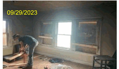
Image Type:Completion During Photo Address:4433 Virginia Ln City,State Zip:Forth Worth, TX 76103 Line Item Desc:Photos
