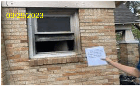
Image Type:Completion Before Photo Address:4433 Virginia Ln City,State Zip:Forth Worth, TX 76103 Line Item Desc:Photos
