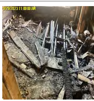
Comp/Insp Date: 9/29/2023 Damage Photo
