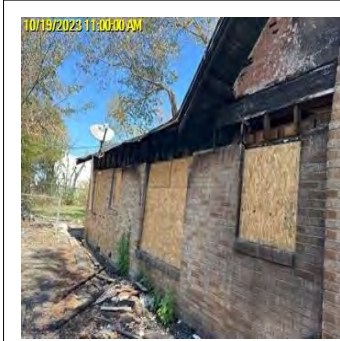
Comp/Insp Date: 10/19/2023 Damage Photo
