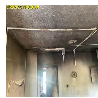
Comp/Insp Date: 9/29/2023 Damage Photo
