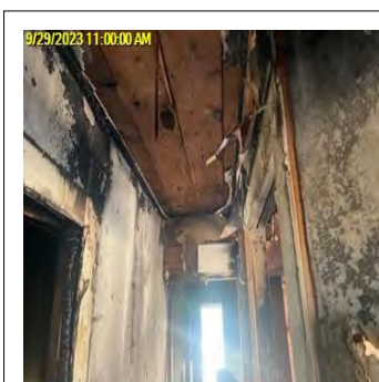
Comp/Insp Date: 9/29/2023 Ceiling - Interior
