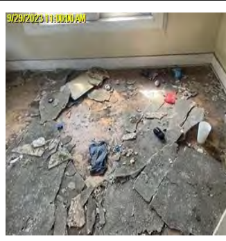
Comp/Insp Date: 9/29/2023 Damage Photo
