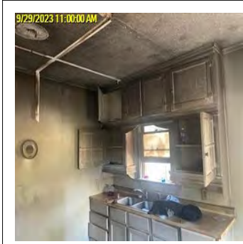
Comp/Insp Date: 9/29/2023 Stove/Oven
