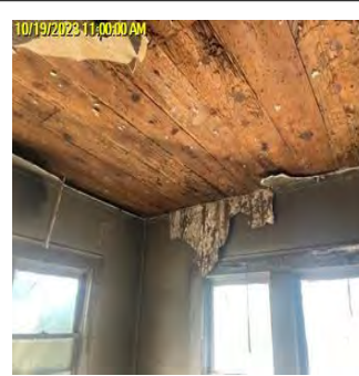
Comp/Insp Date: 10/19/2023 Ceiling - Interior
