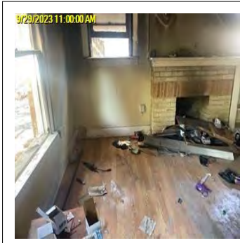
Comp/Insp Date: 9/29/2023 Damage Photo
