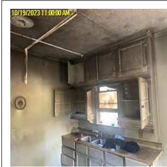
Comp/Insp Date: 10/19/2023 Ceiling - Interior
