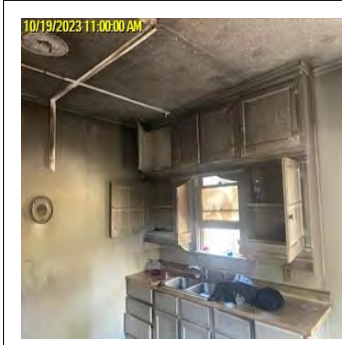
Comp/Insp Date: 10/19/2023 Stove/Oven
