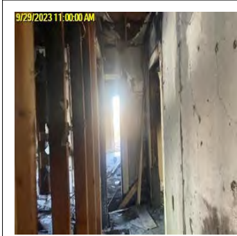
Comp/Insp Date: 9/29/2023 Damage Photo
