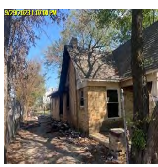
Comp/Insp Date: 9/29/2023 Bid Photo Trim Ex Lg Tree - 39-78in Trunk Diameter & 51-102 ft Tall - Ea addtl Tree - Includes Clean Up of Clippings - Assumes Work Area is Obstacle Free
