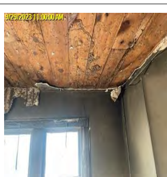
Comp/Insp Date: 9/29/2023 Ceiling - Interior
