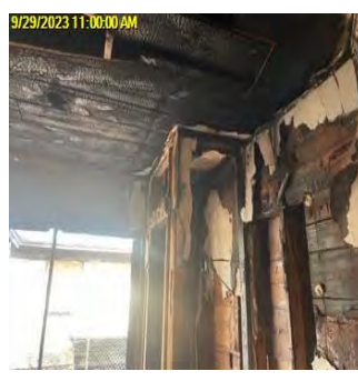
Comp/Insp Date: 9/29/2023 Damage Photo
