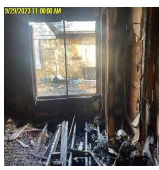
Comp/Insp Date: 9/29/2023 Damage Photo
