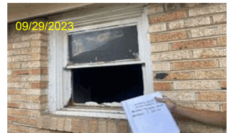
Image Type:Completion Before Photo Address:4433 Virginia Ln City,State Zip:Forth Worth, TX 76103 Line Item Desc:Photos
