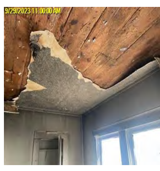
Comp/Insp Date: 9/29/2023 Damage Photo
