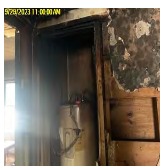
Comp/Insp Date: 9/29/2023 Damage Photo
