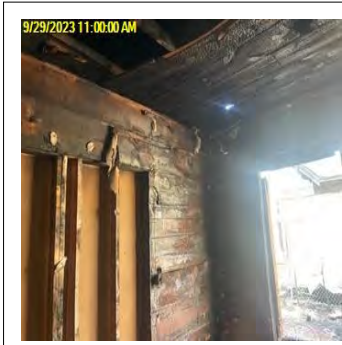
Comp/Insp Date: 9/29/2023 Ceiling - Interior
