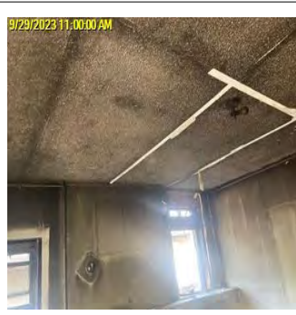
Comp/Insp Date: 9/29/2023 Damage Photo
