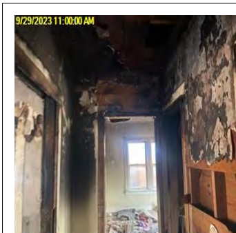
Comp/Insp Date: 9/29/2023 Damage Photo
