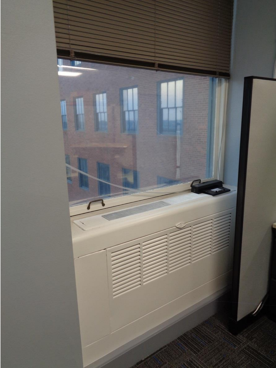
Photo 28: Tenth floor, typical heating/air conditioning unit below historic window; looking southwest.
