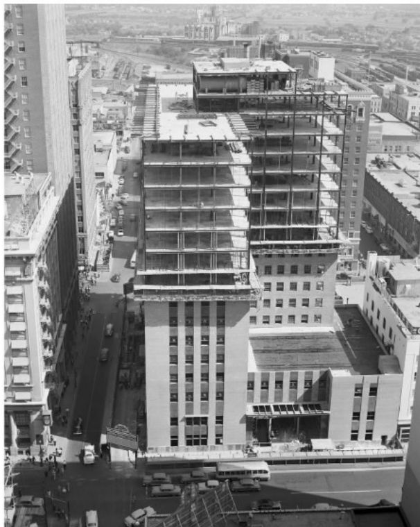
Figure 16 View Exterior of Fort Worth National Bank Building, 1952. East elevation, looking southwest. Courtesy, W. D. Smith Commercial Photography, Inc. Collection, Special Collections, The University of Texas at Arlington Libraries. AR430-52-3-29. Identifier 20097271.
