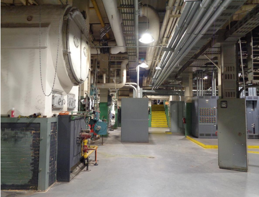
Photo 14: Original boiler (left), sub-basement; looking west.
