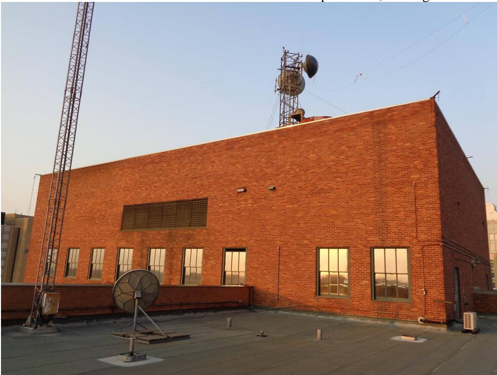
Photo 13: Roof of slab and east and north elevations of penthouse; looking southwest.
