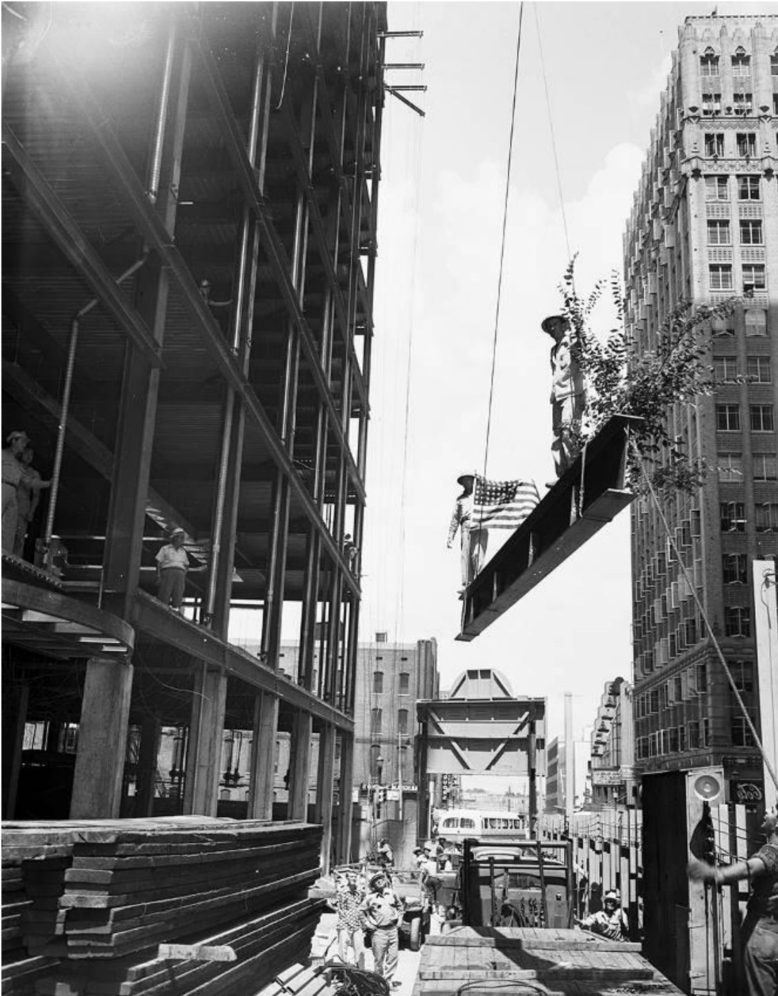
Figure 15: Fort Worth National Bank, 07/31/1951. H. Warren Smith, steel foreman, and Ed Grimes, inspector, ride the beam as the last piece of steel is hoisted into position atop the new Fort Worth National Bank Building. Courtesy, Fort Worth Star-Telegram Collection , Special Collections, The University of Texas at Arlington Libraries. AR406-6-457. Identifier 20126776.
