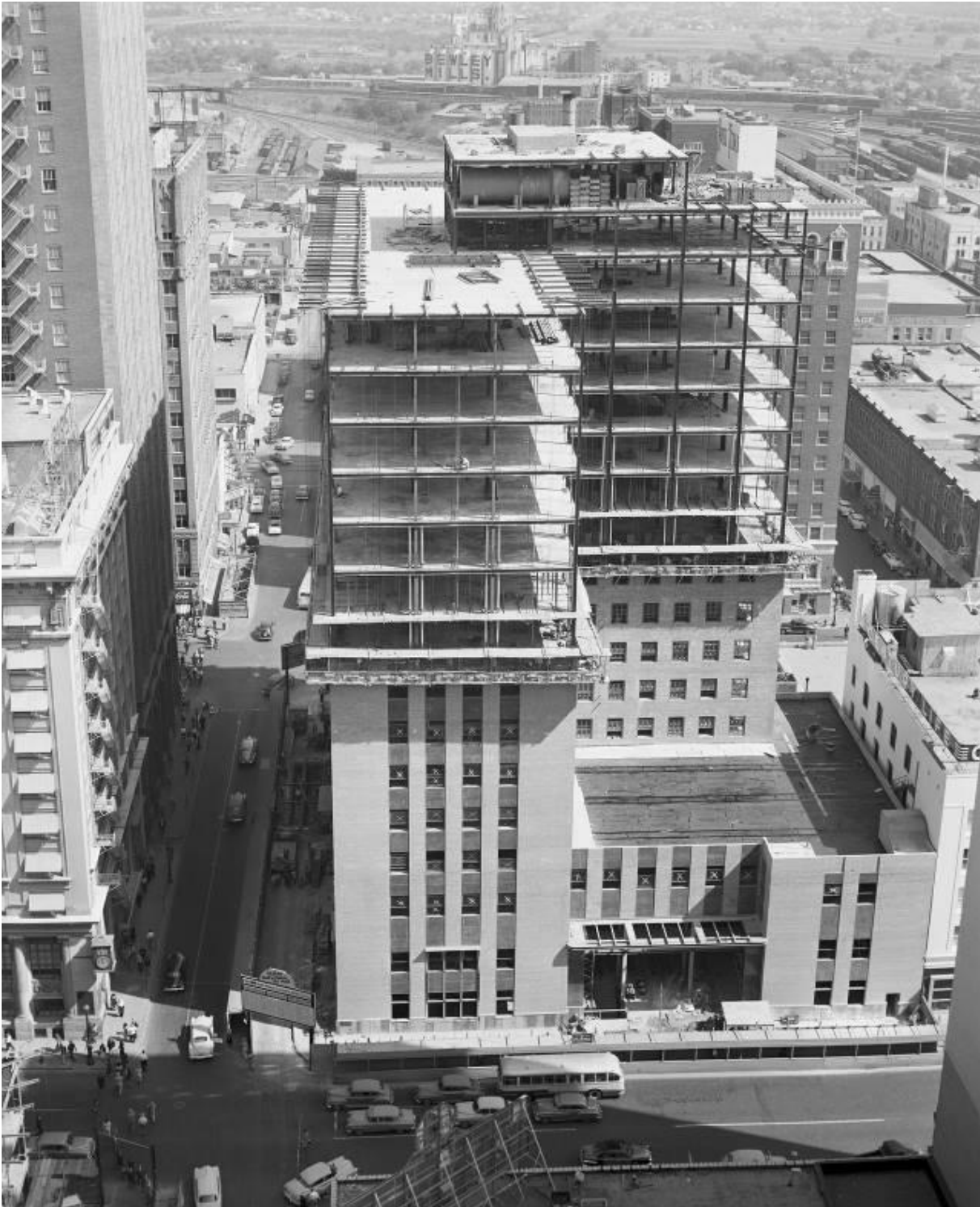
Figure 16: Fort Worth National Bank Building, Construction Progress #97. Looking east. Courtesy, W. D. Smith Commercial Photography, Inc. Collection, Special Collections, The University of Texas at Arlington Libraries. AR430-3-214. Identifier 20096485.
