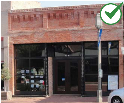
After: Historic storefront elements are exposed, following removal of non-historic stucco and other material.
