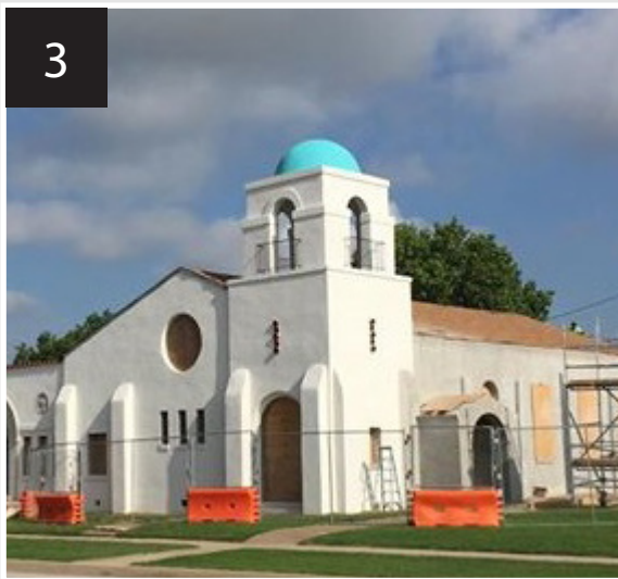
Phase 1 Rehabilitation: Interim improvements to the building included reopening the transom, providing a new sign and reconstructing the kickplate.
