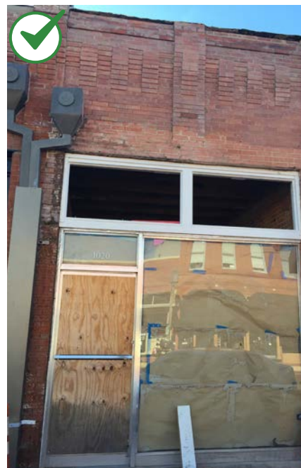
After: Historic material revealed
