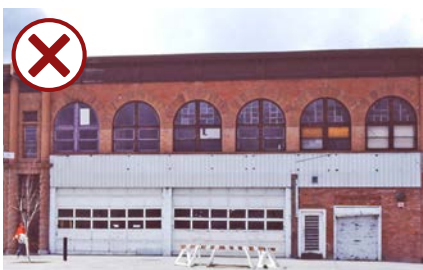
Remodeling the storefront of a historic building (Fort Collins, CO) to accommodate an auto repair shop is inappropriate. Storefronts were removed to make way for a garage. (Compare with the image below.)
