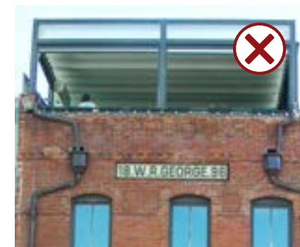
This rooftop deck is set too close to the edge of the historic building wall and impedes one's ability to interpret the historic scale and character of the original structure.
