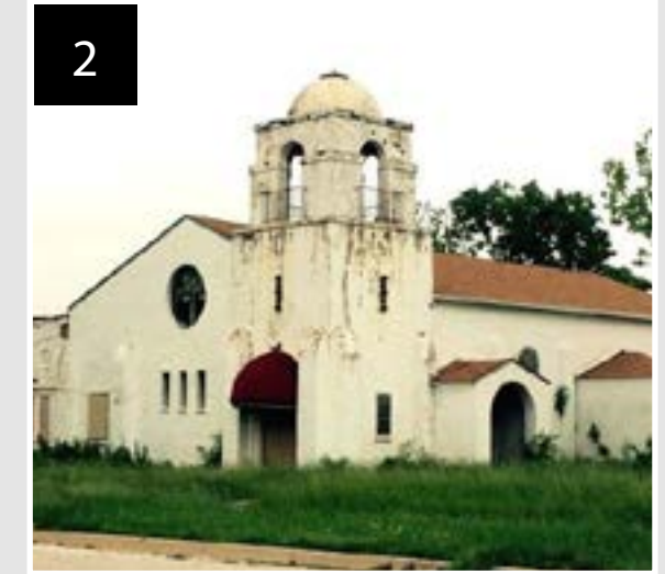
Once scheduled for demolition the building was not maintained and was left abandoned and dilapidated.
