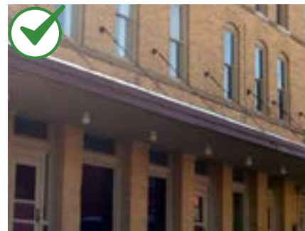
Appropriate canopy supporting mechanisms are wall mounted brackets, cable suspended columns or chains consistent with the style of the building.
