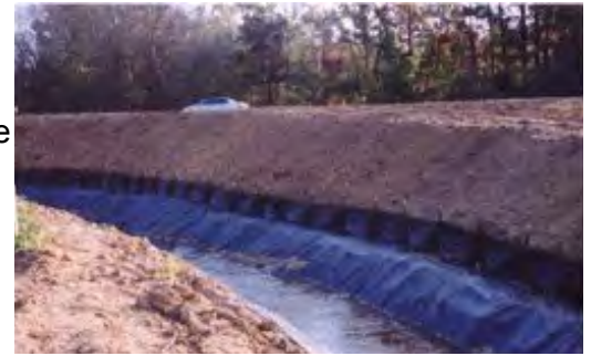
Figure 7.10-9: Fabric Lined Diversion Channel
