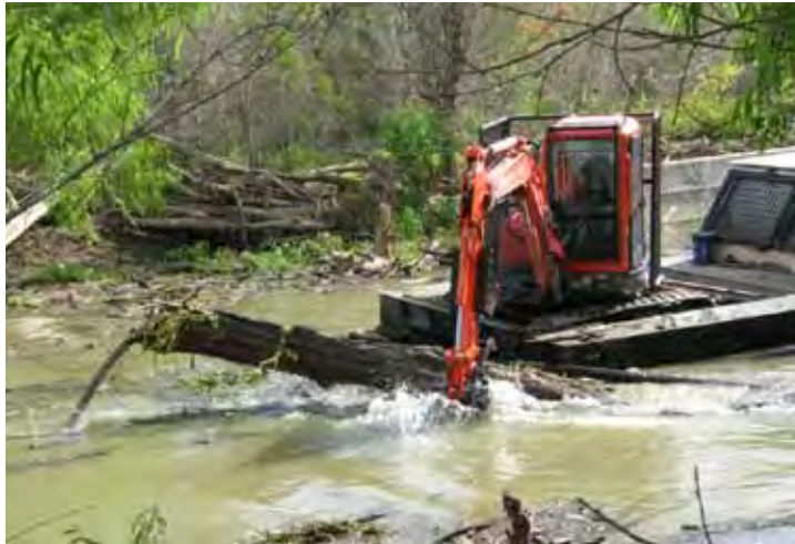
Log Jam Removal Operations on the San Antonio River in Refugio County, TX
