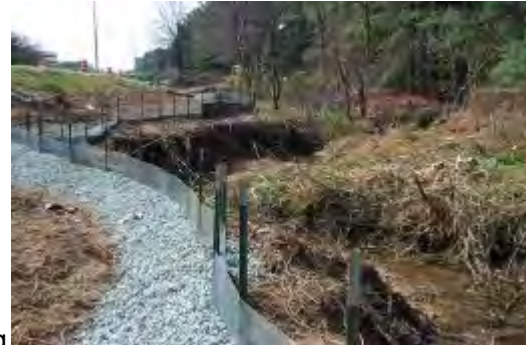
Figure 7.10-4: Sediment Control Fence
