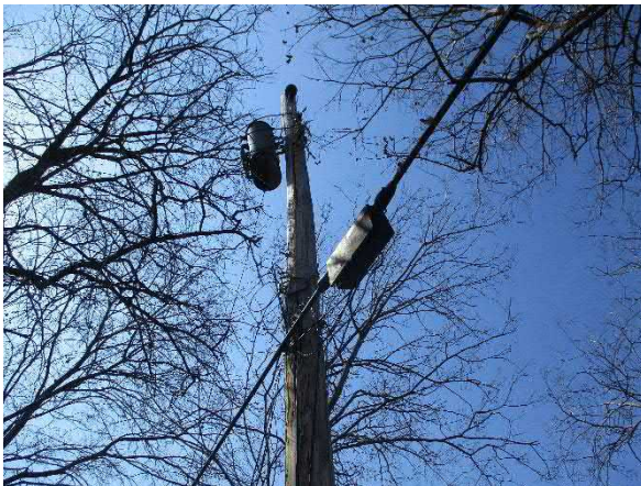
Photo #9 Representative view of the pole-mounted transformers located throughout the site.
