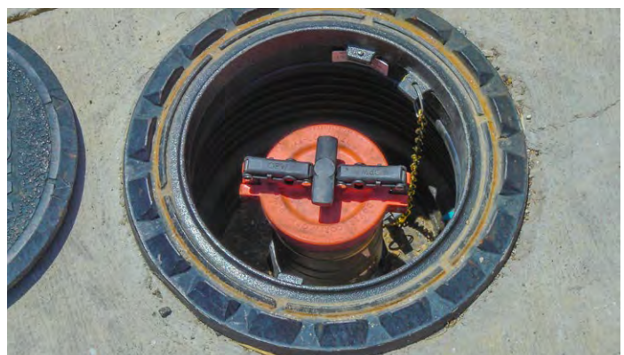
Figure 5-22. Environmental staff must inspect fuel ports on USTs to verify tank compliance, photo by City of Fort Worth.
