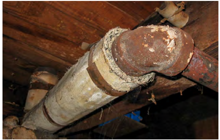
Figure 5-13. A pipe insulated with asbestos-containing materials, photo by City of Fort Worth.
