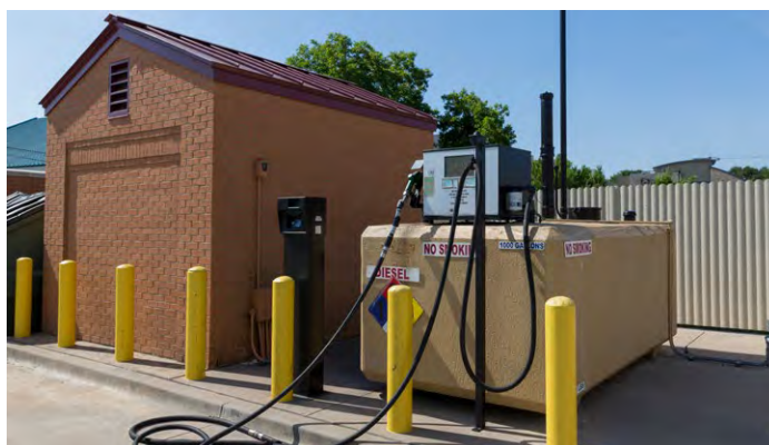
Figure 5-21. Environmental compliance is critical for ASTs like this fuel tank at a FWFD fire station, photo by City of Fort Worth.
