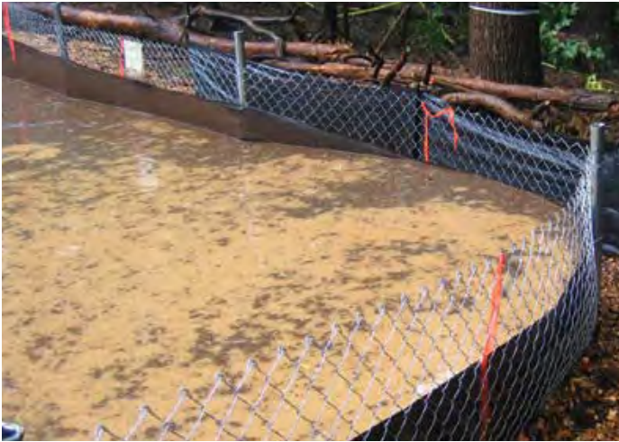
Figure 4-25. A silt fence with a chain link support is used on a construction site to prevent stormwater pollution, photo from EPA.
