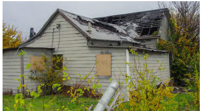
Figure 2-17. A substandard structure that has been damaged by fire, photo by City of Fort Worth.
