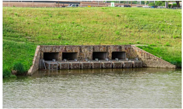
Figure 6-14. This TRWD trash basket traps debris and allows water to pass through, photo by City of Fort Worth.
