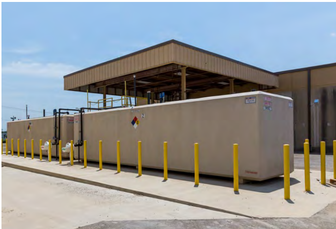
Figure 5-9. A reinforced AST has replaced a leaking UST at a city facility, photo by City of Fort Worth.
