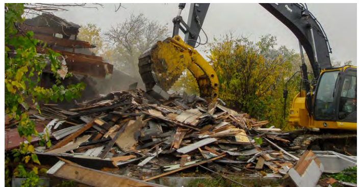
Figure 2-18. The substandard structure pictured above is demolished, photo by City of Fort Worth.
