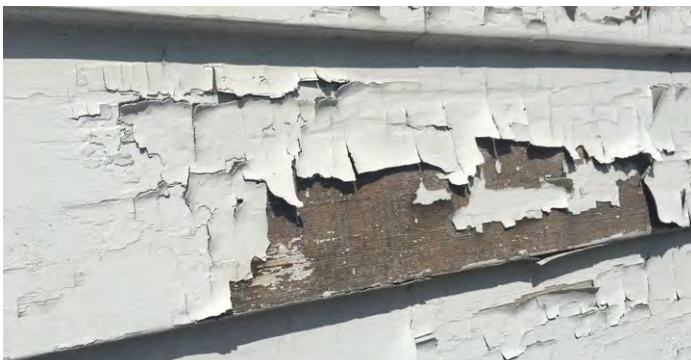
Figure 5-5. Peeling lead paint on the siding of a substandard structure, photo by Mike Mozart.
