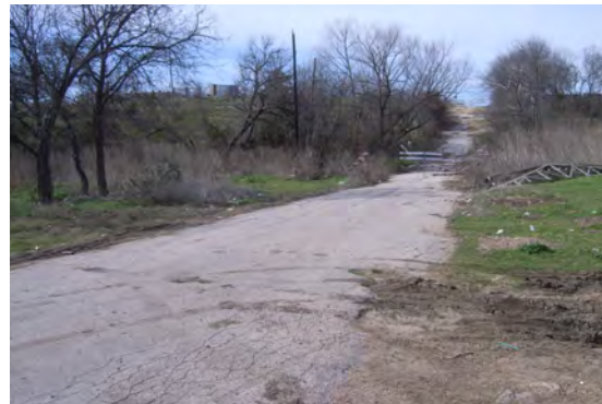
Unimproved poor condition street in Como.
