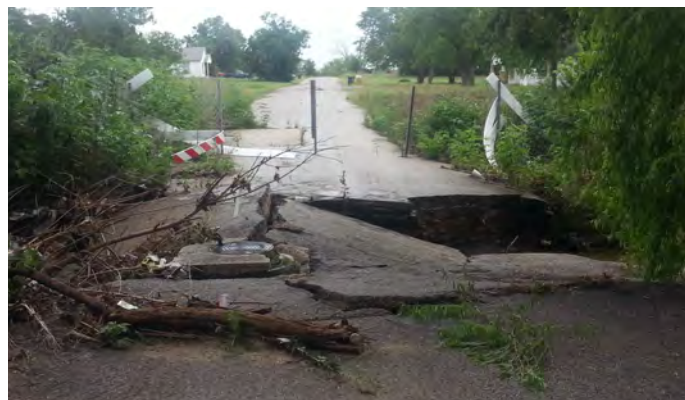
A segment of Farnsworth Street is closed due to recurrent flooding that exceeded the underground storm drain's capacity, resulting in a caved in street.
