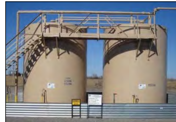
Typical storage tanks
