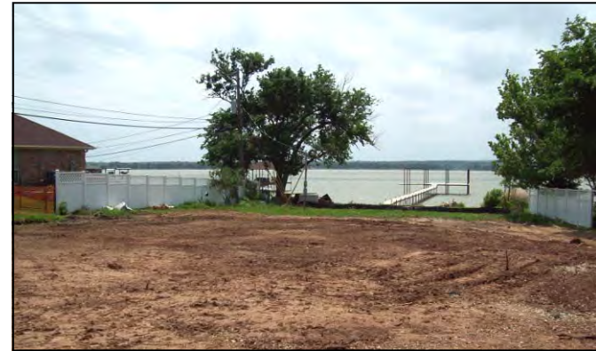
New development on Lake Worth; silt fence in place; grass buffer good aid in catching silt runoff
