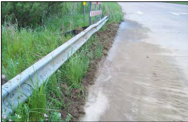
Sediment that has made it through silt fences north of Loop 820/South of Jacksboro Highway
