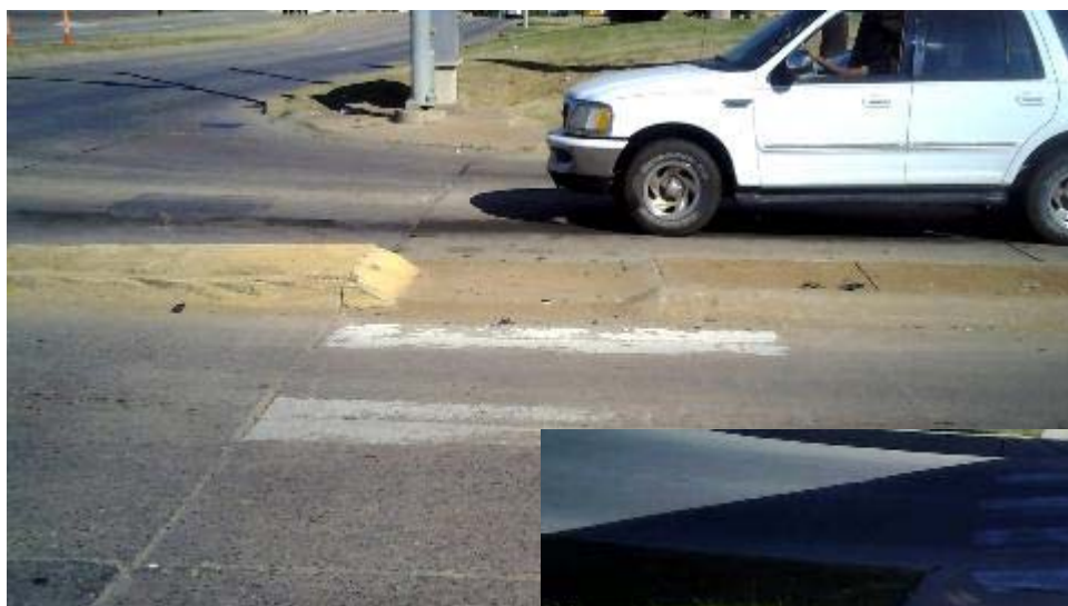
Non-compliant: Sides not 90°
