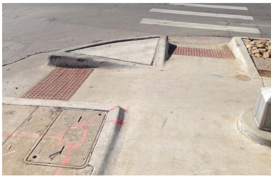
NON-COMPLIANT (traversable adjacent surface)
