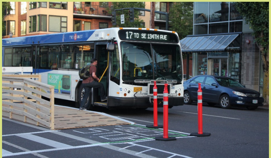
A line of bright green tape was added along the edge for visibility purposes, and skid-resistant tape was secured to the island ramps.
