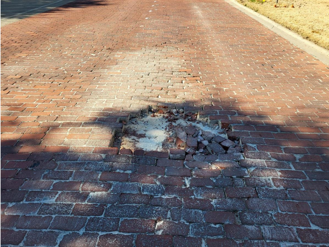
Deteriorated Concrete Base and Brick Pavement
