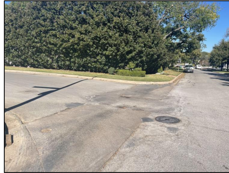
Damaged valley gutter
