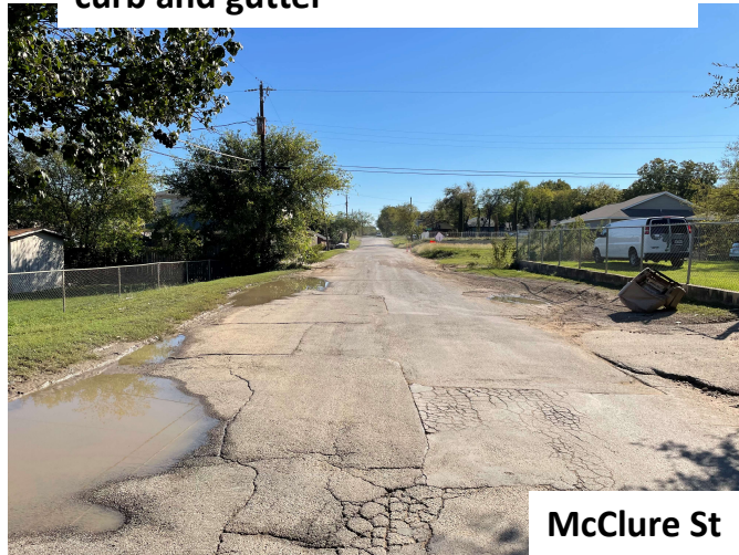
Damaged Asphalt Paving, missing curb and gutter
