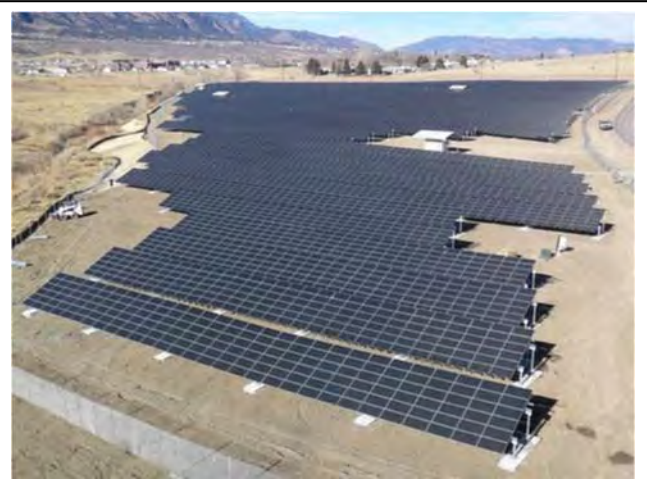
A PV System on a closed landfill near Atlanta Georgia. Source: Feasibility Study of Economics and Performance of Solar Photovoltaics at the Vincent Mullins Landfill in Tucson, AZ.
