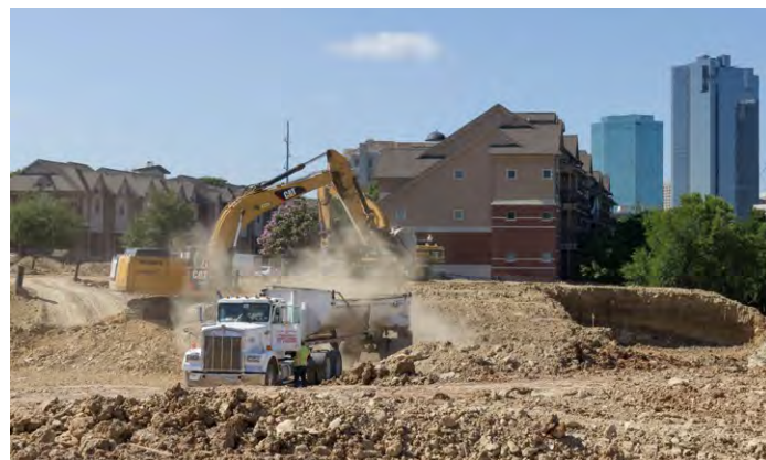
Figure 3-24. Dust blowing from activity on a construction site. If too much dust is generated and escapes the site, it can lead to enforcement action, photo by City of Fort Worth.
