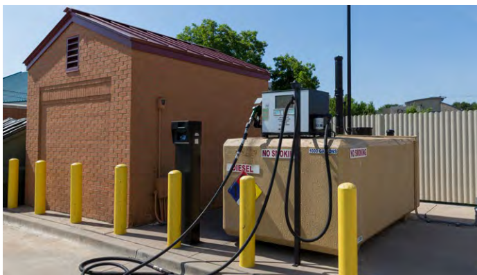
Figure 5-21. Environmental compliance is critical for ASTs like this fuel tank at a FWFD fire station, photo by City of Fort Worth.
