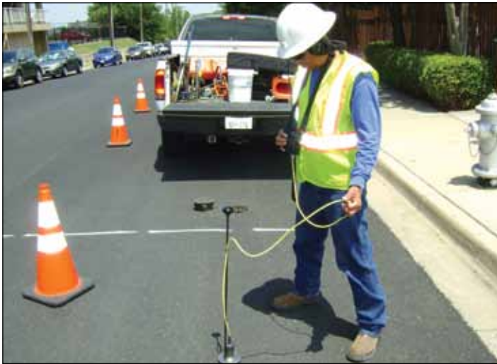
A trained employee uses special equipment to listen for leaks on buried water lines.
